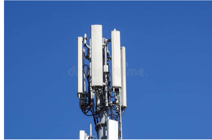
4G mast with sectoral antennas
